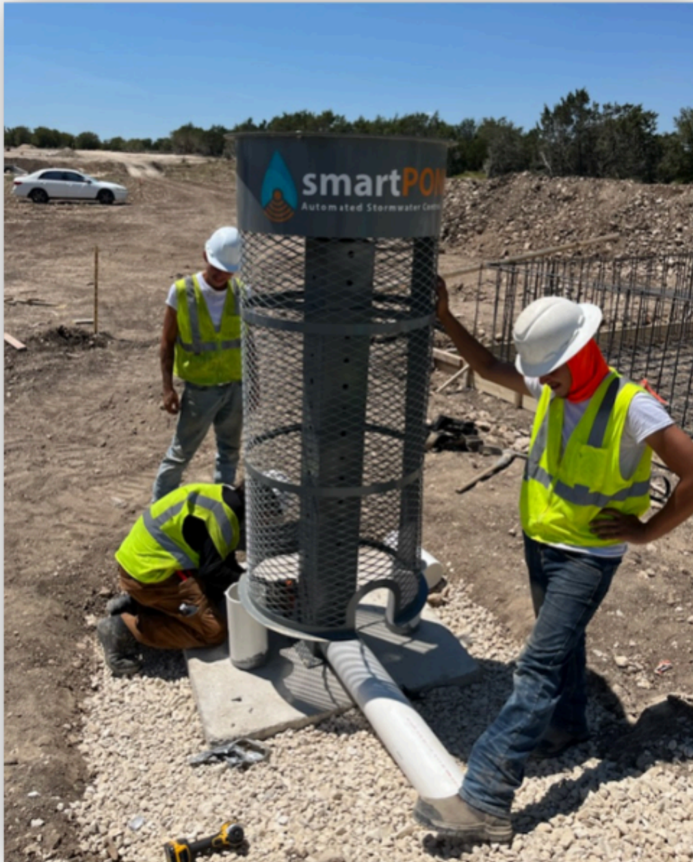
6. Attach the discharge pipe to the inlet screen riser and route to location of the valve assembly
